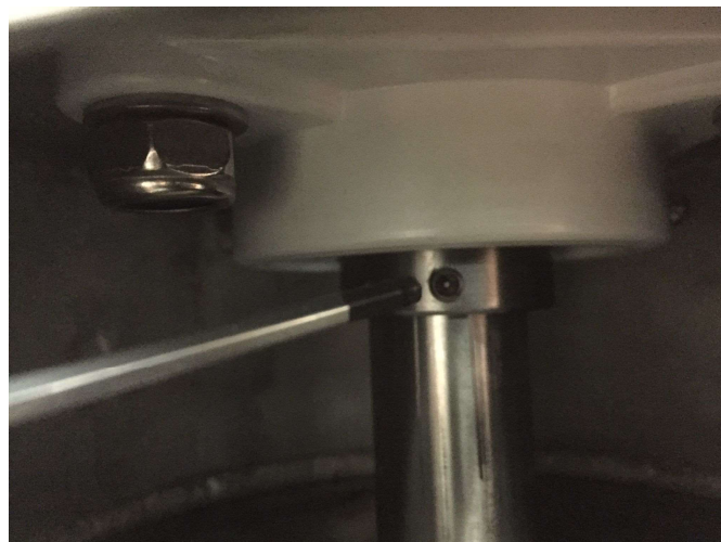
Figure 12: Close-up of the bearing through the inspection window. There are two Allen head (size 3) screws that fixate the shaft in the bearing.
